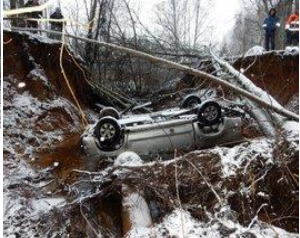
Water washed dam, bridge and road in Antsla Community 15.10.2015 after beavers blocked overflow
